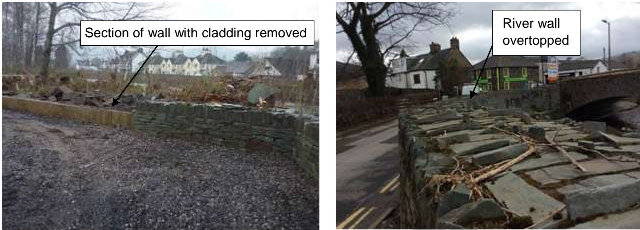
Figure 27 River overtopped its bank/flood wall at Southey Hill Estate and the river wall overtopped at upstream of Greta Bridge
