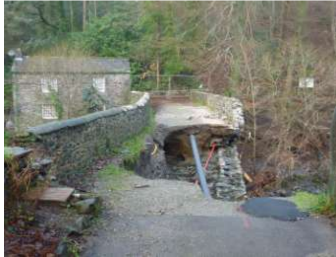
Figure 13 Forge Bridge Partially Collapsed
