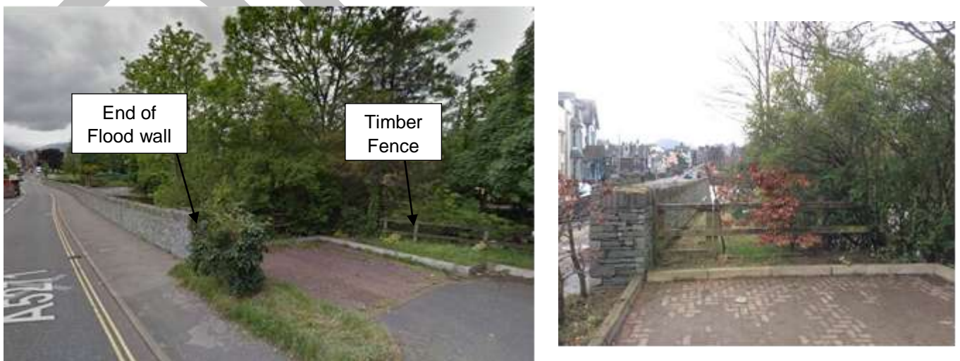
Figure 19 Left bank of River Greta where defences overtopped
