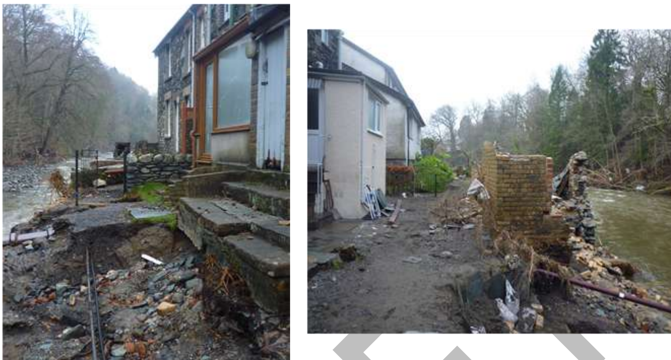
Figure 15 Scour damage to the rear of properties
