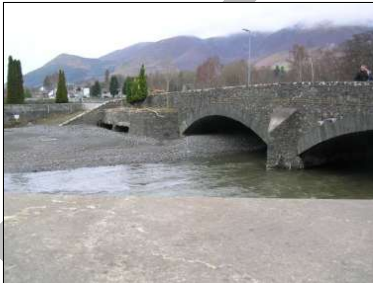
Figure 8 Blockage of culverts downstream of Greta Bridge
