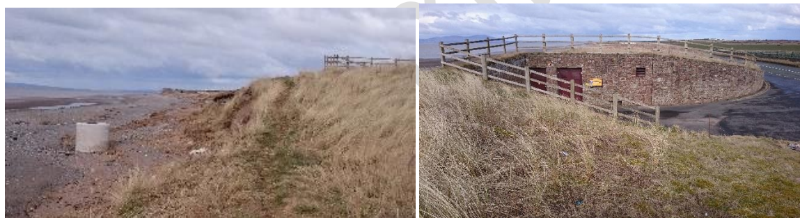
Figure 7 United Utilities Pumping Station in eroded dune frontage south of Crossbeck. Photographs taken February 2018.
