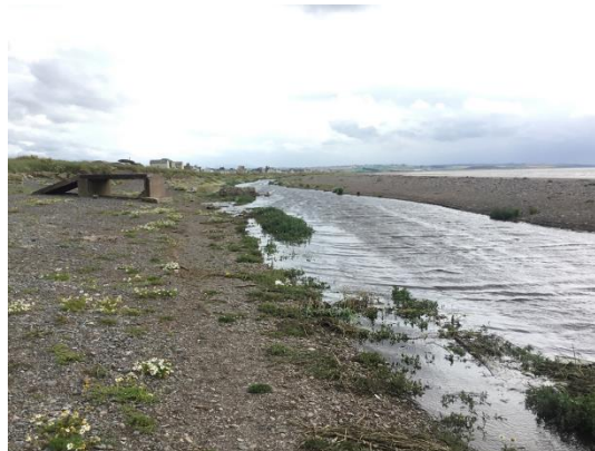
Figure 6 Allonby frontage: the beck is diverted northwards by a shingle spit. Photograph taken during CH2M (2017) asset inspection.
