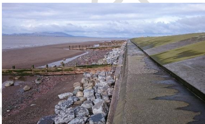
Figure 12 Revetment and seawall at Dubmill Scar. Rock armour was placed along the toe in 2010. Photograph taken February 2018.
