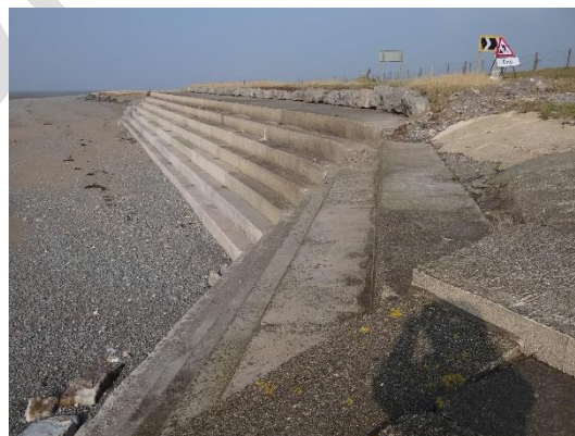
Figure 16 Crest of seawall South of Dubmill Point. Photograph taken during CEUK asset inspection (March 2015).
