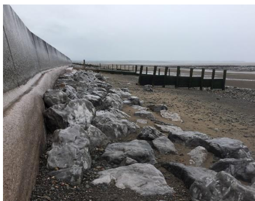
Figure 11 Revetment and seawall at Dubmill Scar. Rock armour was placed along the toe in 2010. Photograph taken August 2017.
