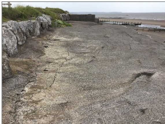
Figure 3 Dubmill Point: armour stone wall. Photograph taken during CH2M (2017a) asset inspection.
