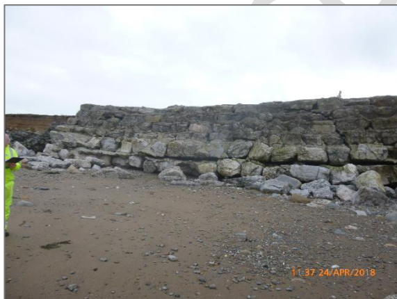
Figure 5 Dubmill Point: armour stone wall front elevation. Photograph taken during CCC Inspection (Apr 2018).
