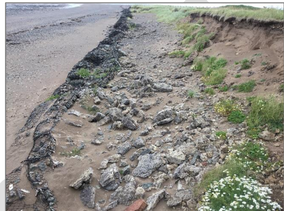
Figure 4 Gabion baskets at Dubmill Point – there is evidence of erosion along the backshore, suggesting the effectiveness of this defences has diminished over time.
