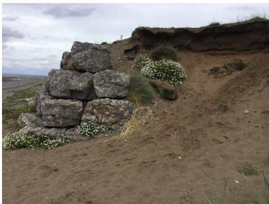
Figure 7 Rock armour wall south of Beckfoot. Terminal erosion is evident. Photograph taken during CH2M (2017a) asset inspection.
