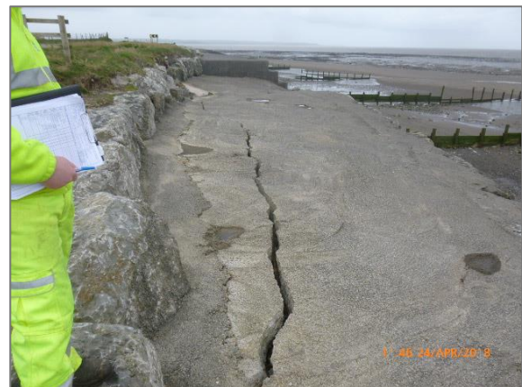
Figure 6 Dubmill Point: armour stone wall crest – movement of wall. Photograph taken during CCC Inspection (Apr 2018)
