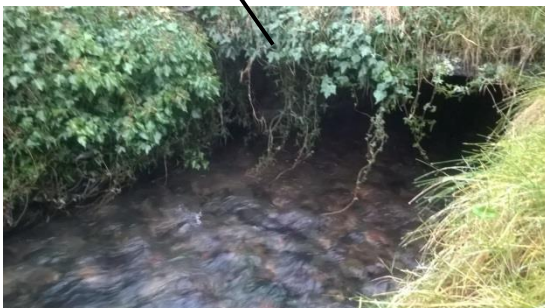
Culvert outfall into Holme Beck at village Hall. 450mm x 450mm brick. Flows well.
