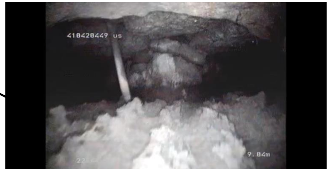
Junction (looking in upstream direction). The flow from Hillside comes through the right branch which is 300mm x 300mm stone.
