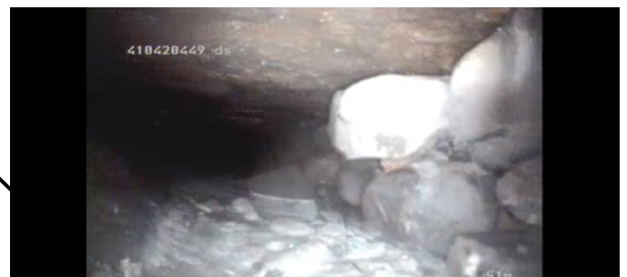
Debris shoal restricts clearance and camera can't get through. Walls crumbling in. Where good the shape is approx. 450mm w x 300mm d stone.
