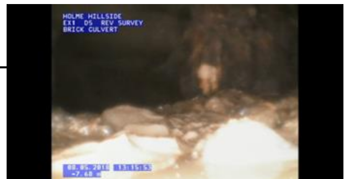
Cannot be sure if there is a split to the right (looking downstream) here.
