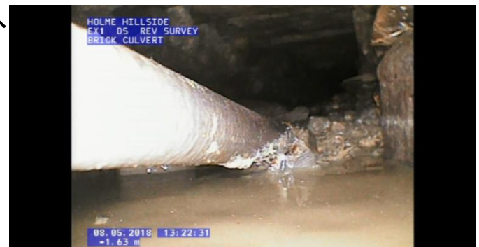
Survey ends here, just beyond the fence line, where collapse is near total and there is an unidentified pipe within the culvert barrel. No further progress with camera in downstream direction. Significant flow does come through as proven by dye testing.
