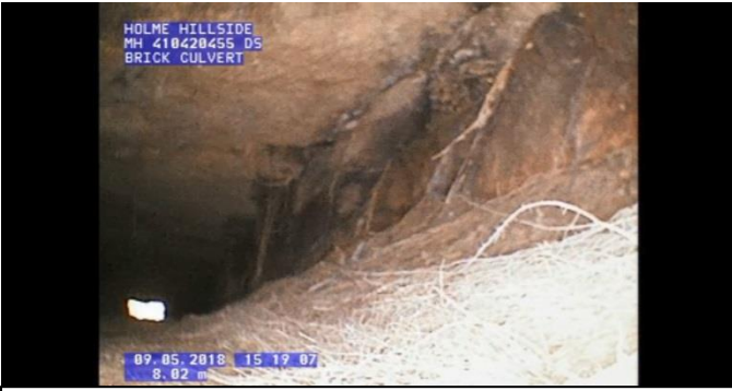
Camera caught in roots. Daylight visible downstream. 450mm x 450mm, brick.
