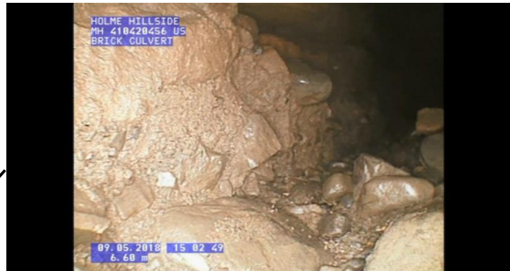
Stone debris restricts clearance deflects camera into sides. Camera can't get through.
