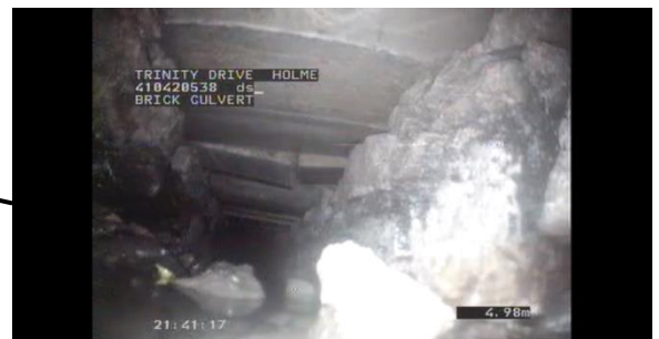
Walls tilting inwards preventing passage of camera. 450mm x 450mm, brick.
