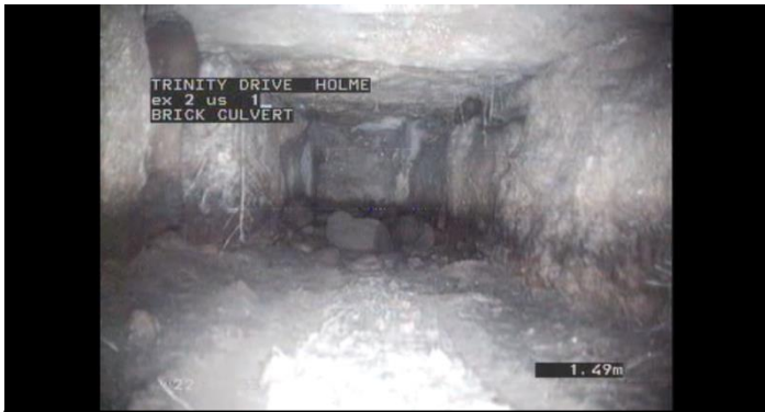
The left branch looking upstream is either capped off or has collapsed directly beneath the wall of the building. The dimensions are 300mm x 300mm stone.
