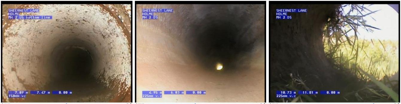
Figure 16: Images from CCTV survey along Sheernest Cottages back alley to northernmost outfall drainage run.
