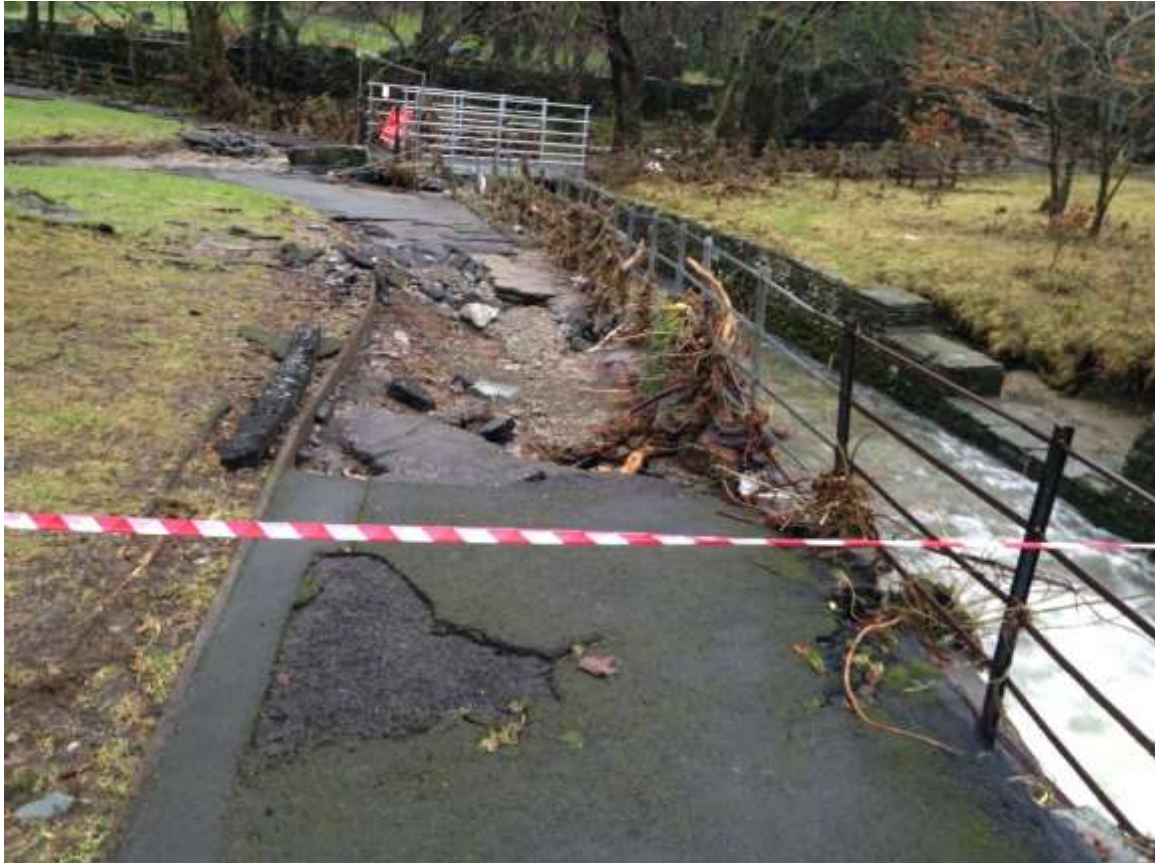
Figure 18 - Flood damage caused to a footpath by Stock Ghyll in Rothay Park. Note the level of the debris in the railings.
