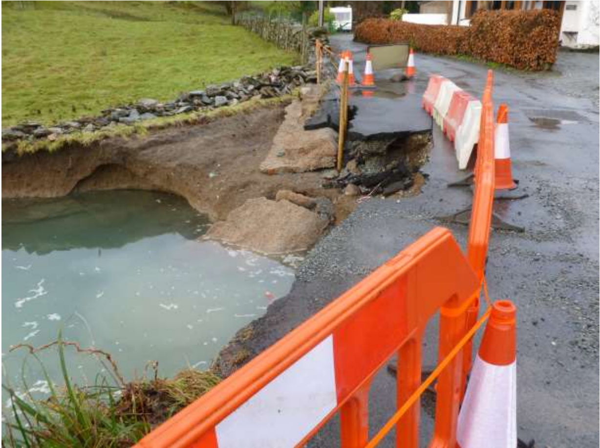
Figure 27 - Flood damage by River Rothay on Under Loughrigg Road
