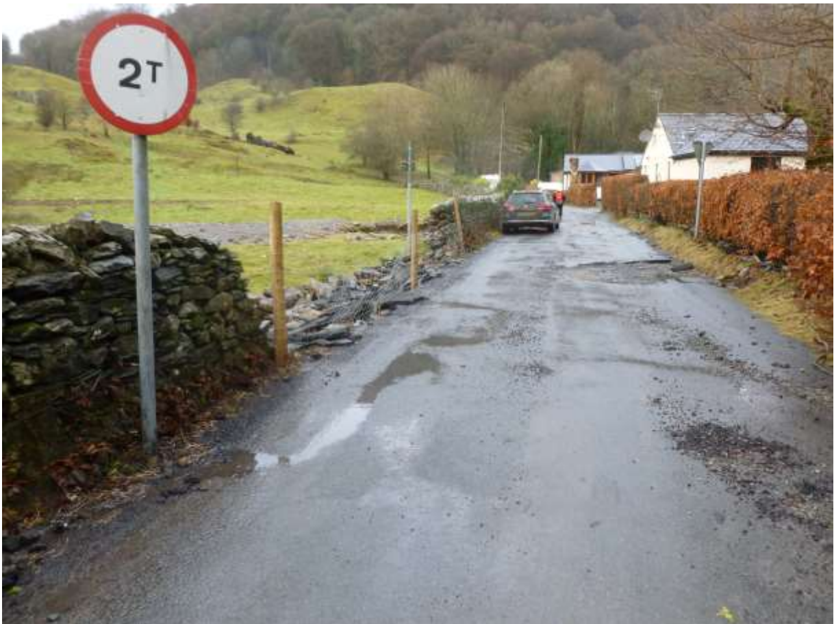
Figure 28 - Flood damage by River Rothay on Under Loughrigg Road
