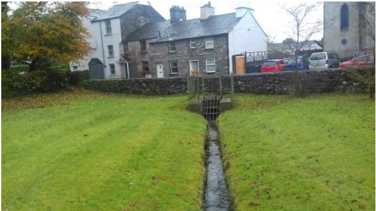
Figure 14 – Culvert inlet on Greenbank Ghyll, just upstream of Rydal Road and opposite cottages shown in Figure 15
