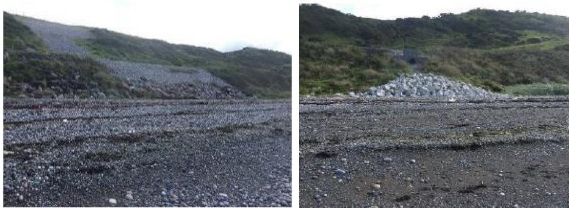
Figure 12 11d5.5 to 11d5.6 random tipped protection to the railway embankment. Rock shown in right photo appears to act as a spillway to a minor culvert.
