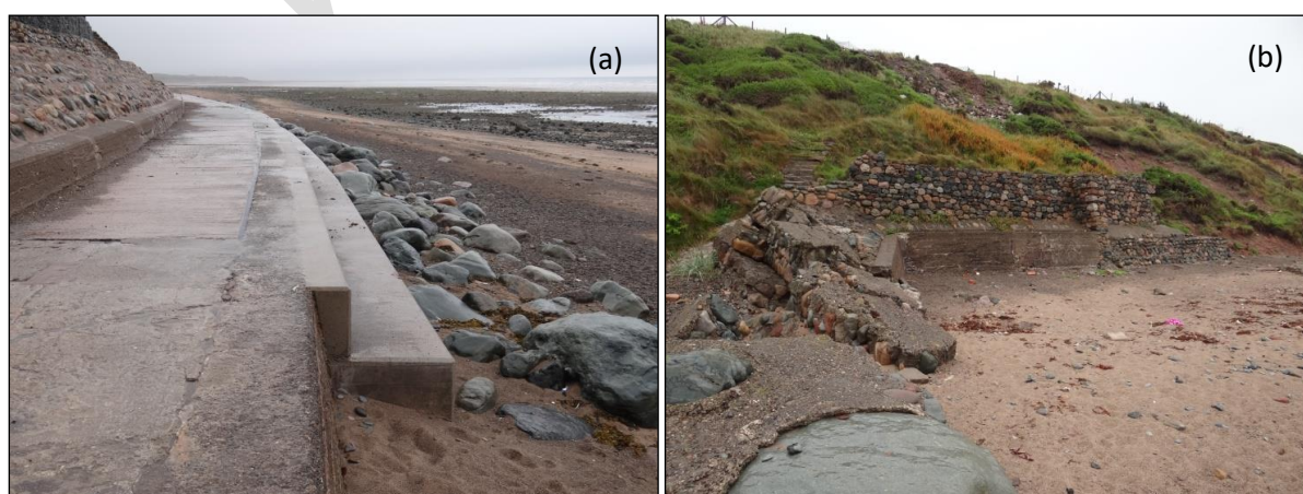
Figure 3 (a) Seascale concrete seawall (b) South of Seascale masonry wall (Site visit photo 2015; CEUK, 2016)
