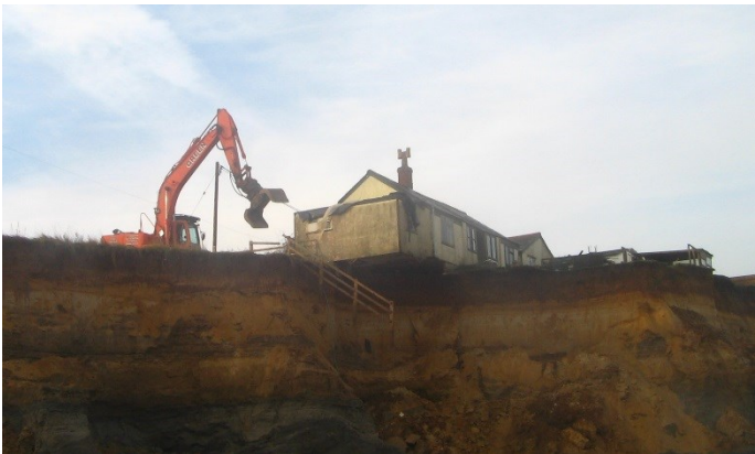
Figure 12: A property at risk of coastal erosion being demolished (image courtesy of North Norfolk District Council)
